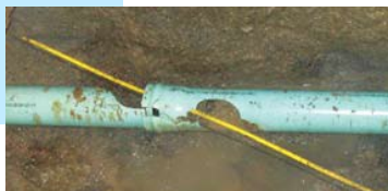
Lateral that has been intersected by a gas line.
